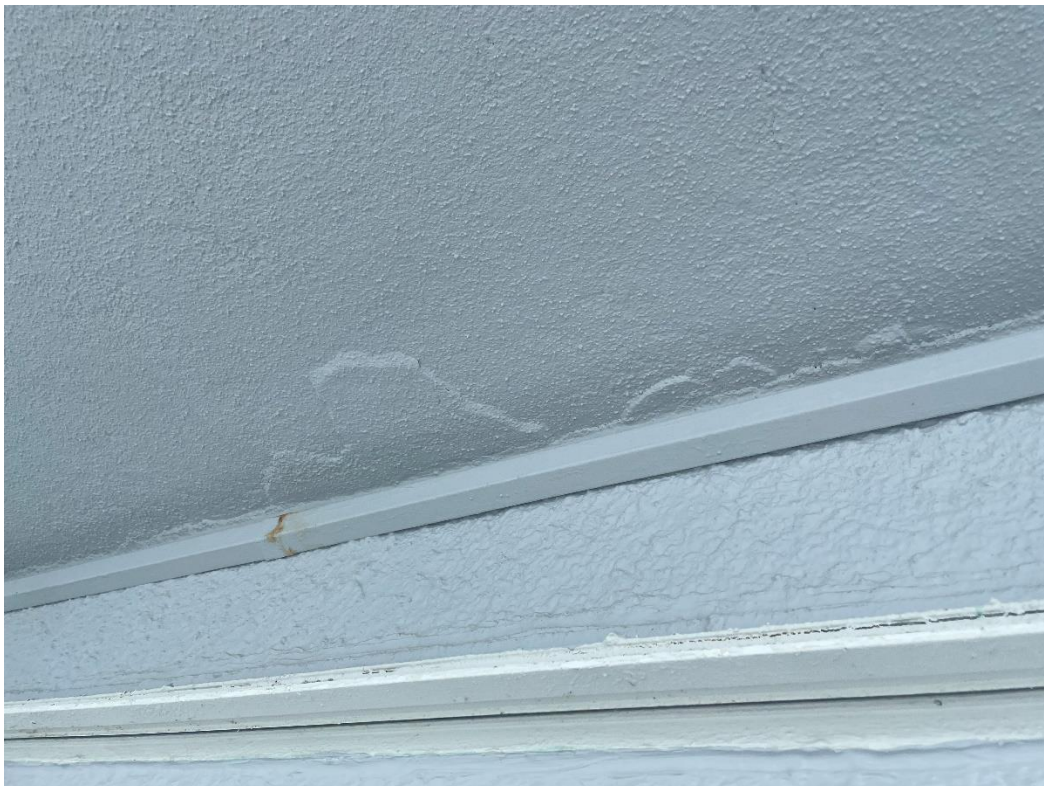
Photo #10 - Overhead Spall
