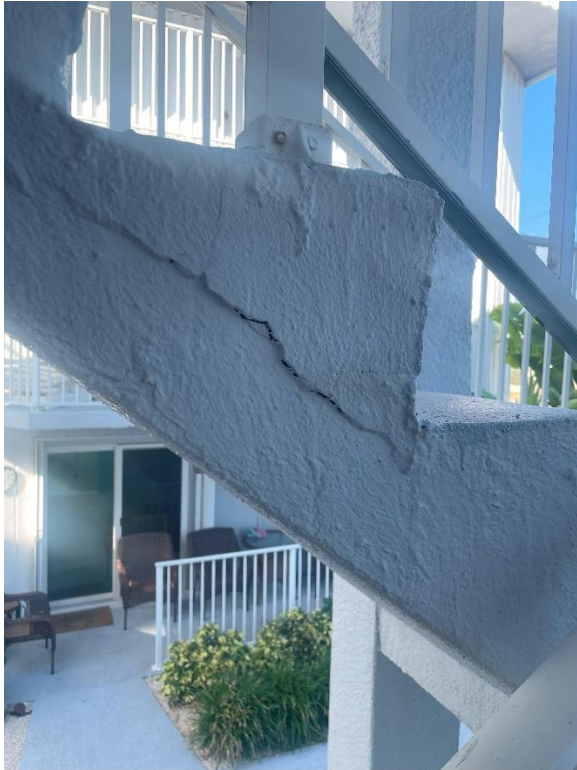
Photo #11 - Spalled Stair Edge
