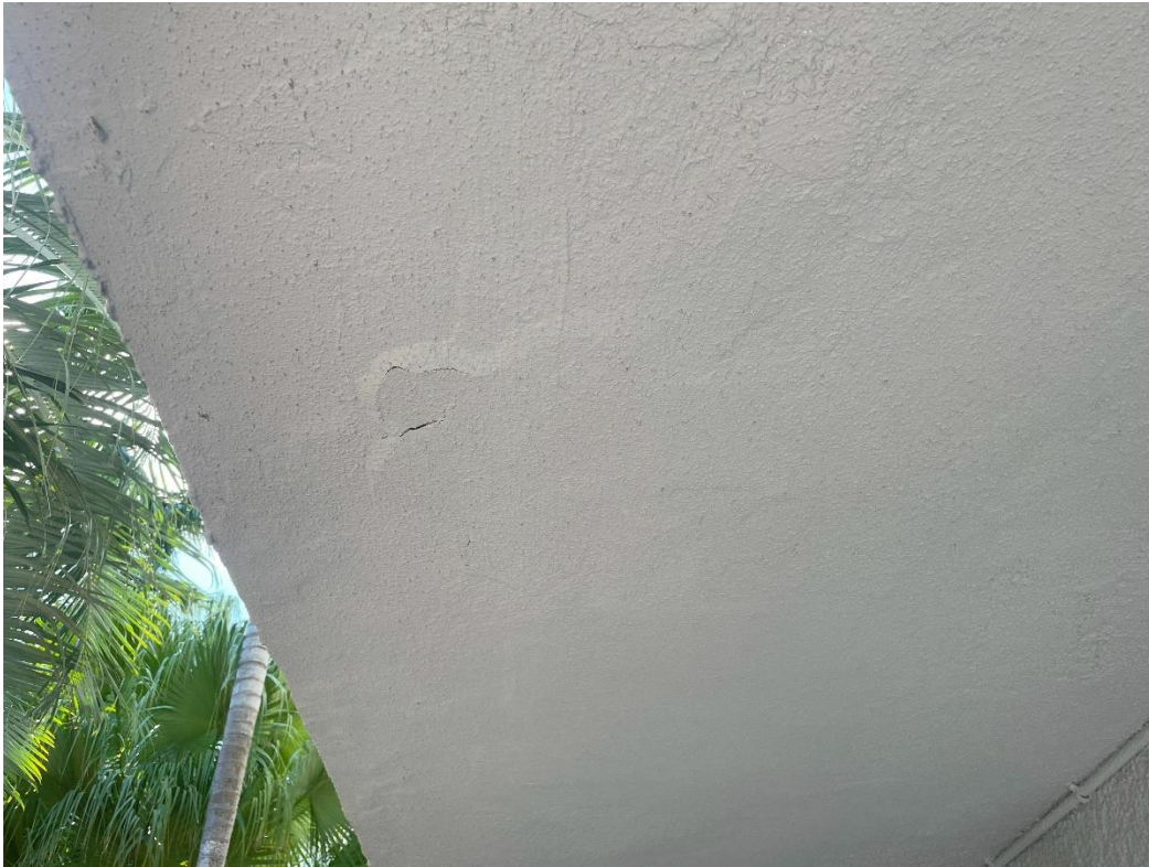
Photo #9 - Overhead Spall
