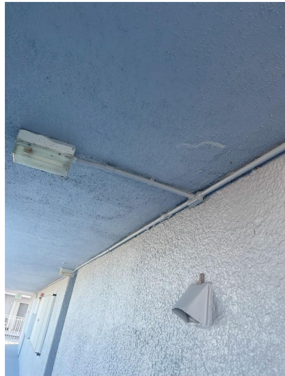
Photo #12 - Overhead Spall
