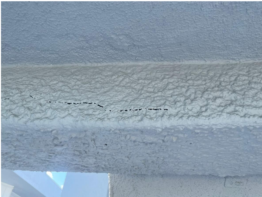
Photo #8 - Crack in Beam
